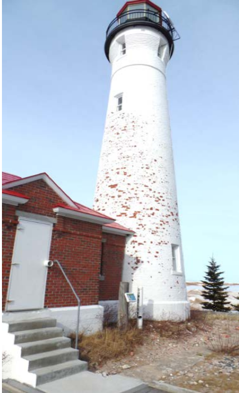
Deteriorating Tower Brick
