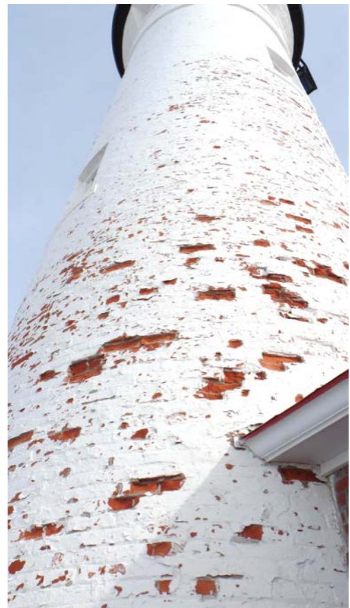
Close up of Deteriorating Tower Brick
