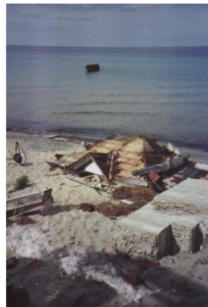
The above picture is of the service building roof lost in November of 1996.
