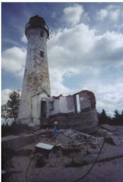
Service building after beach erosion washed out the foundation. This picture was taken in the spring of 1997.
